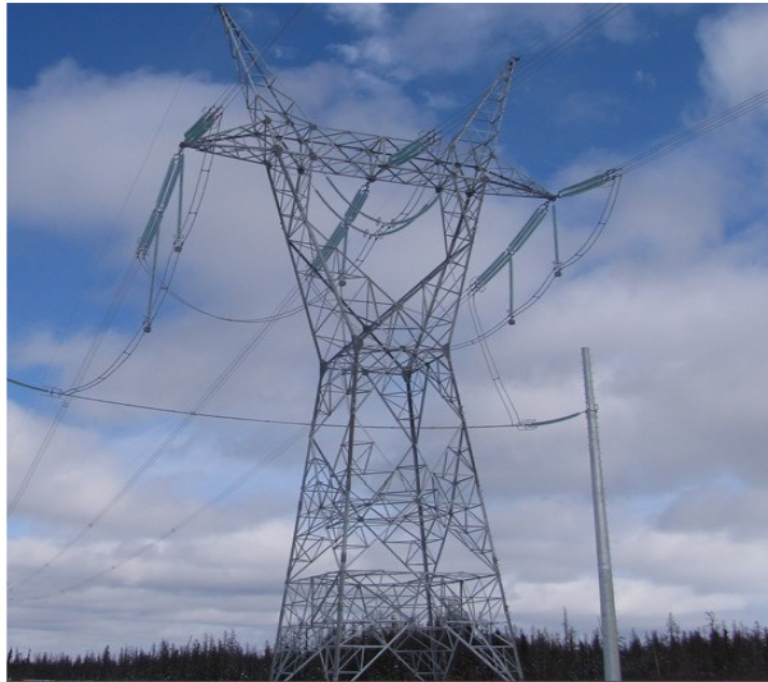
FORT MCMURRAY WEST 500 KV TRANSMISSION
