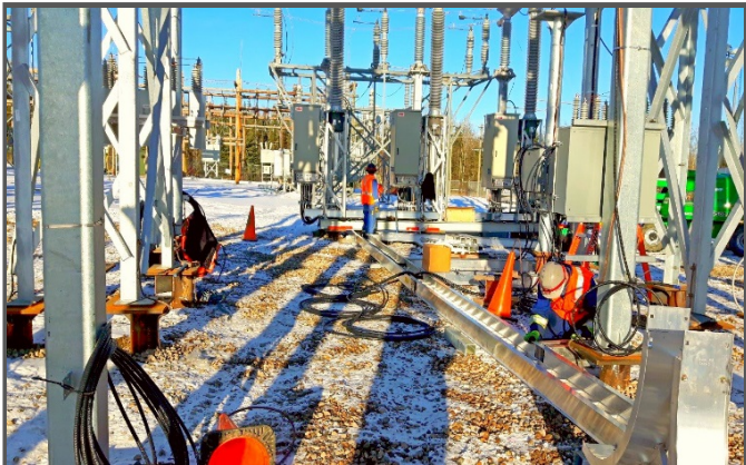
ELECTRIC TRANSMISSION $211M
