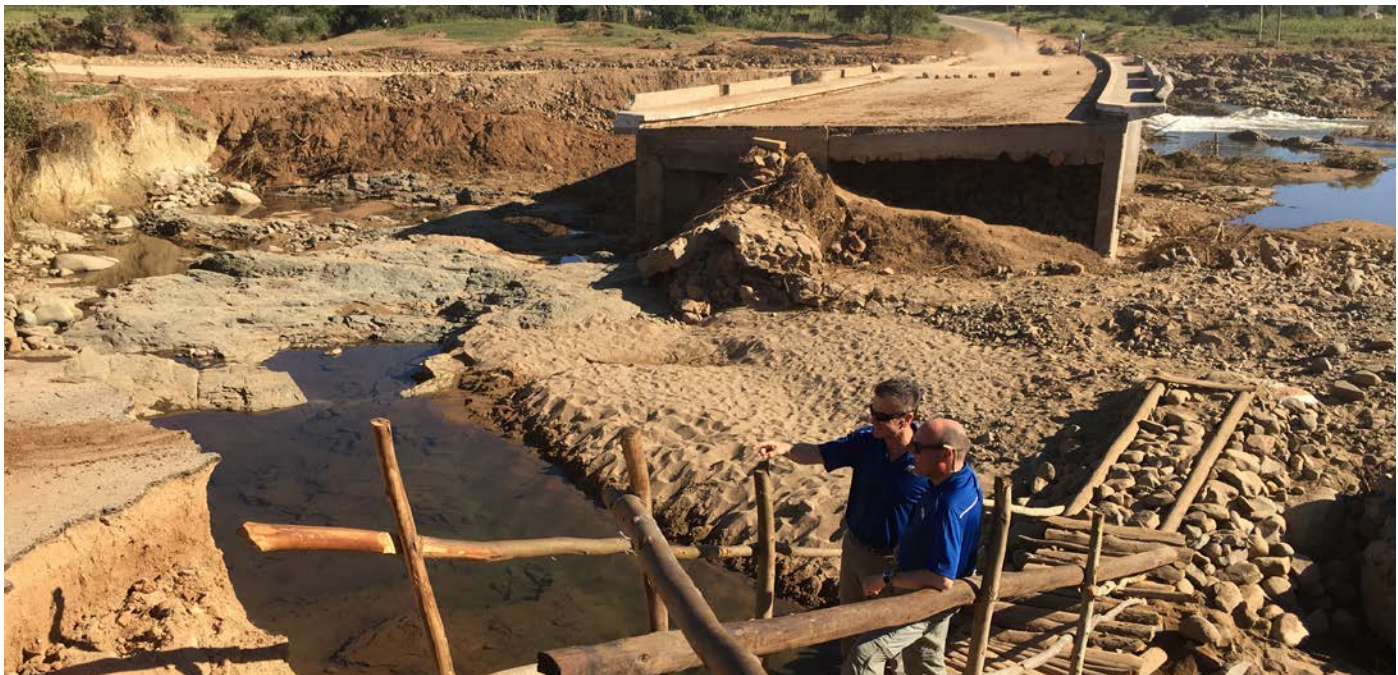
ATCO Frontec employees assess a bridge after Cyclone Idai destroyed it in Zimbabwe, Africa.
