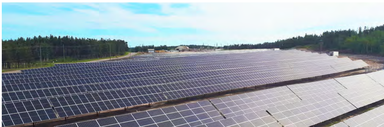
Fort Chipewyan Solar Project, Fort Chipewyan, Alberta
