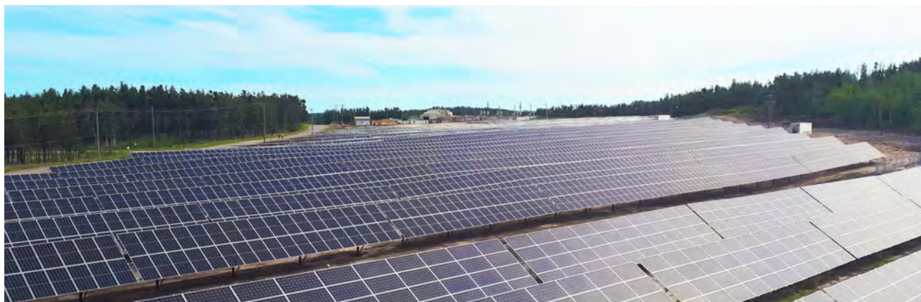
Fort Chipewyan Solar Project, Fort Chipewyan, Alberta
