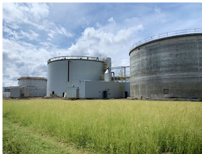
Two Hills Renewable Natural Gas (RNG) Facility - Vegreville, AB
