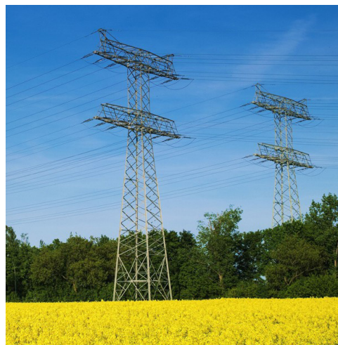
Electricity Transmission Lines
