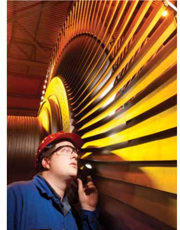
At ATCO Power's 760 megawatt Sheerness generating station, steam turbine blades are inspected as part of regularly scheduled maintenance to ensure maximum efficiency and continued safe, reliable operations of the facility.
